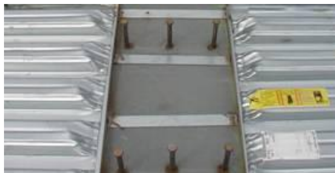
Figure 19 Photograph showing SIP forms attached to a top flange in a tension region
