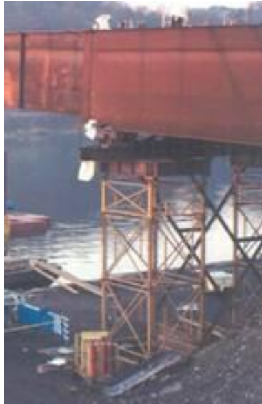
Figure 7 Photograph of a temporary bent
