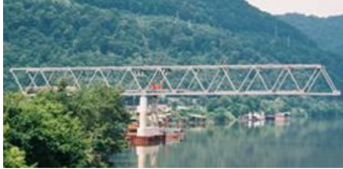
Figure 13 Photograph showing cantilever erection of a continuous truss using barge mounted cranes
