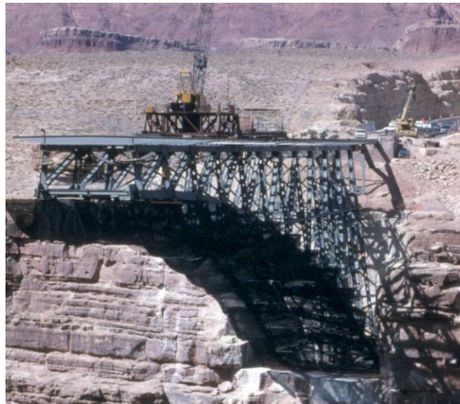
Figure 16 Photograph of an arch bridge erection using the floor system as an erection tie to the canyon wall
