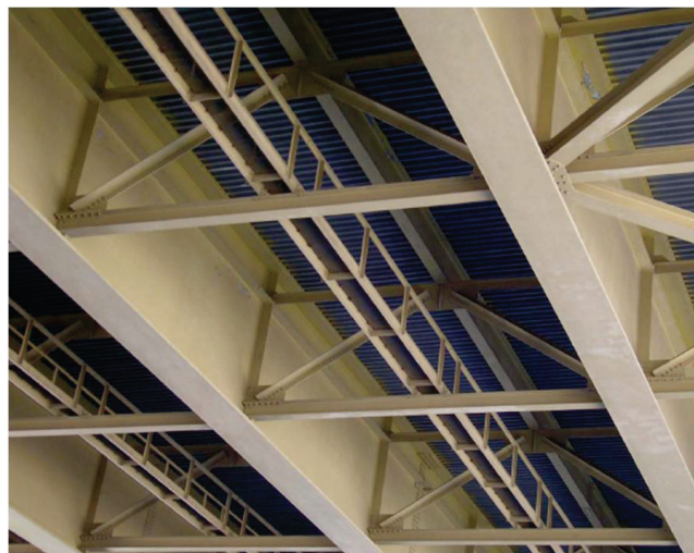
Figure 2 Photo of a typical girder substringer system showing a stringer sitting on top of cross frames
