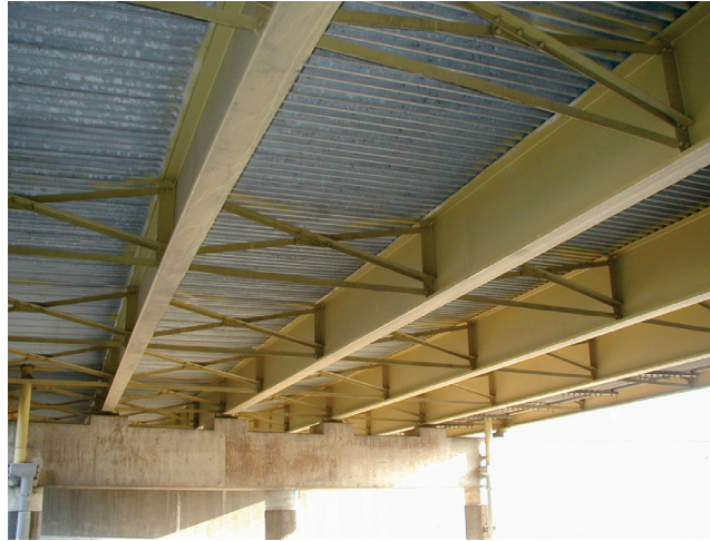
Figure 1 Photo of a typical multi girder system with x-type intermediate cross frames and stay-in-place formwork used for constructing the deck slab
