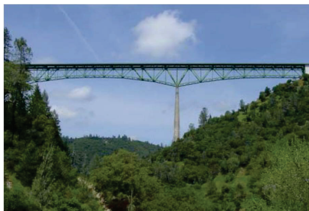
Figure 3 Photo of the Forrest Hill Bridge over American River's north fork, Auburn, California
