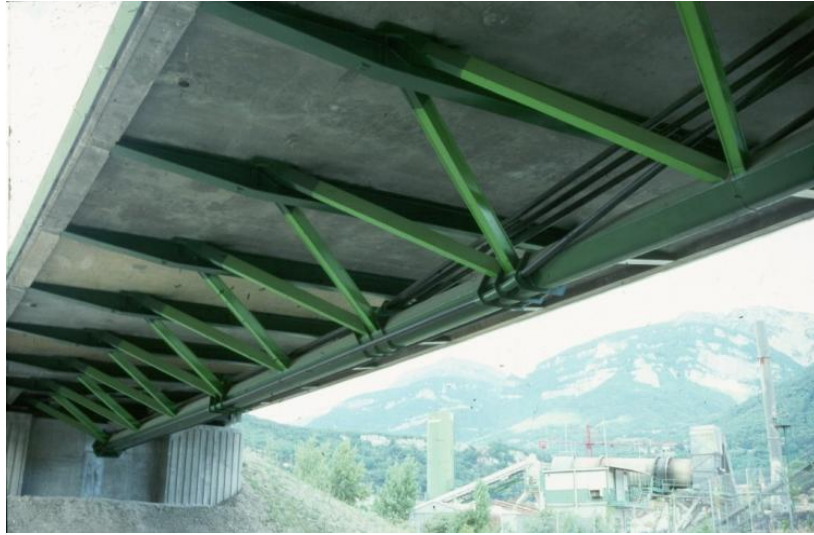
Figure 28 La Roize Bridge in France, triangular cross-section geometry using a single member bottom chord and post-tensioning strand (courtesy of HNTB).
