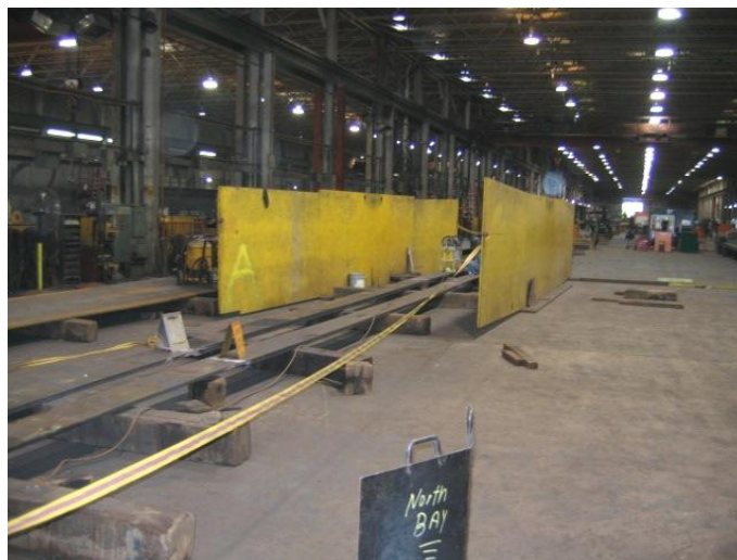
Figure 1 Photo showing the radiographic testing (RT) of a complete joint penetration weld (CJP) with clear area and shielding provided
