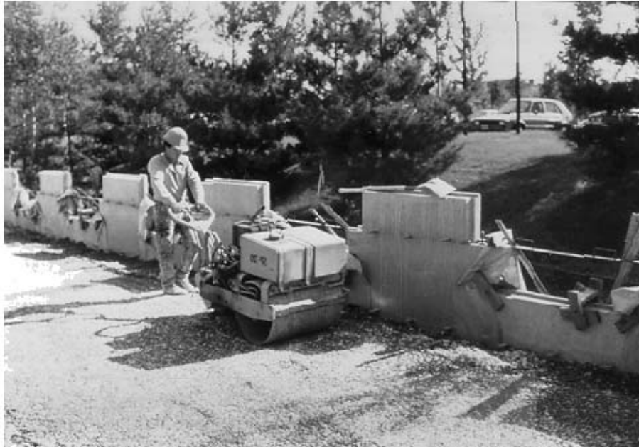
Figure 11-8. Compaction equipment showing: a) large equipment permitted away from face; and b) lightweight equipment within 3 ft (1 m) of the face.
