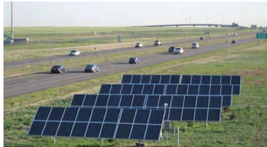
E-470 solar array.
