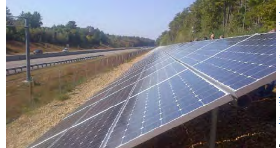
MassDOT solar project along Route 44.
