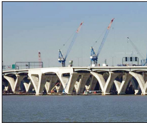
The Woodrow Wilson Bridge is a major project in the Washington, DC, metropolitan area.
