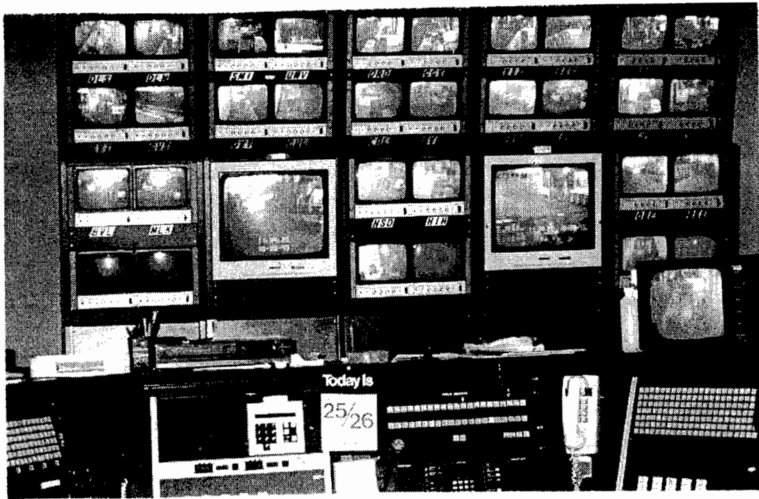
Exhibit 2. Surveillance Monitors at MDTA's Control Center
