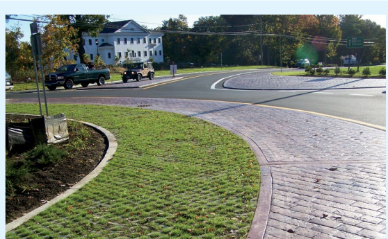
After: Close-up of truck apron constructed during conversion to roundabout, along with a raised truck “blister” on the outside of the roundabout.
