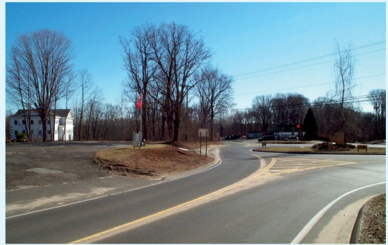
Before: Rotary prior to conversion. Note lack of deflection from entrance on far side of the photo.
