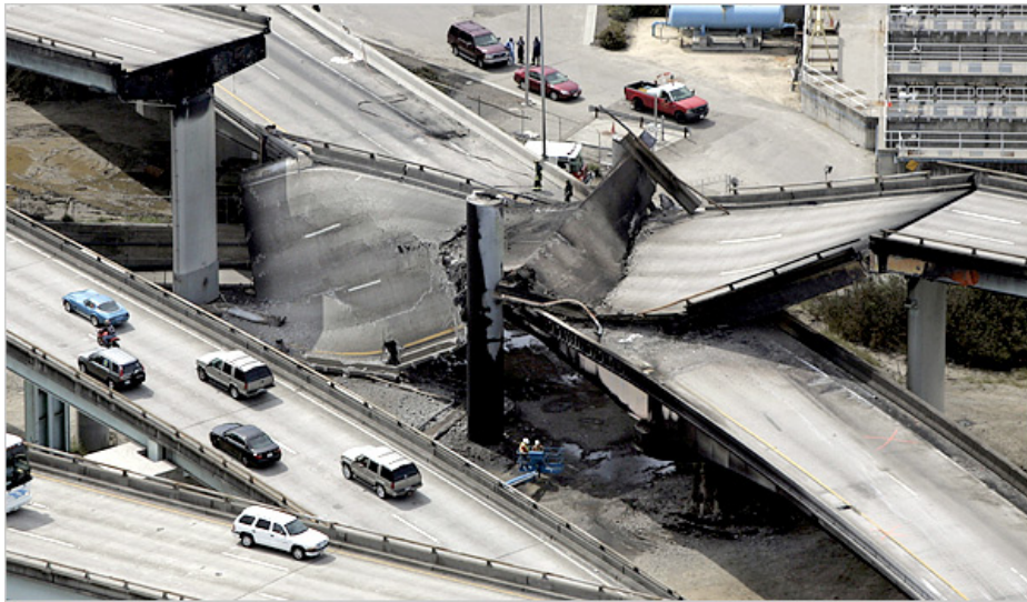
Figure 2.12 I-580 bridge fire (46)
