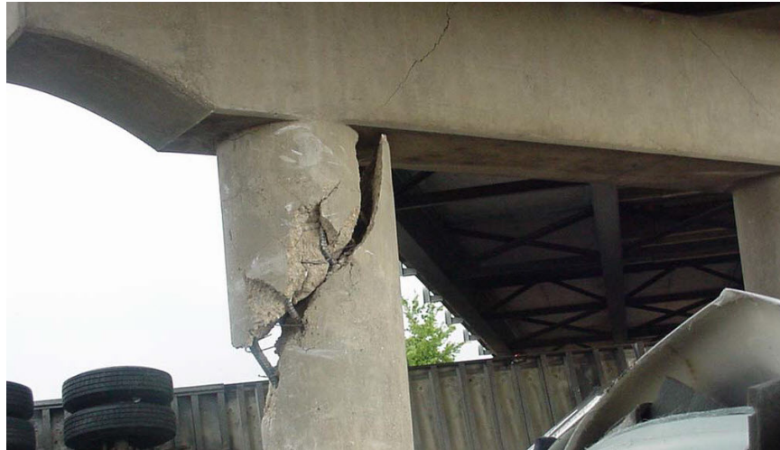
(b) Column failure mode
