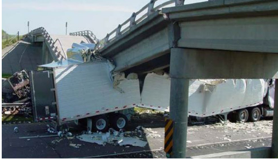
(a) Truck collision with RC column
