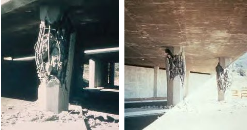
Figure 3.2 Shear failure of a bridge damaged in the 1971 San Fernando Earthquake due to the low thickness and high spacing of the transverse reinforcement (Caltrans 2006).
