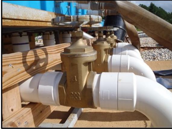
(a) gate valves
