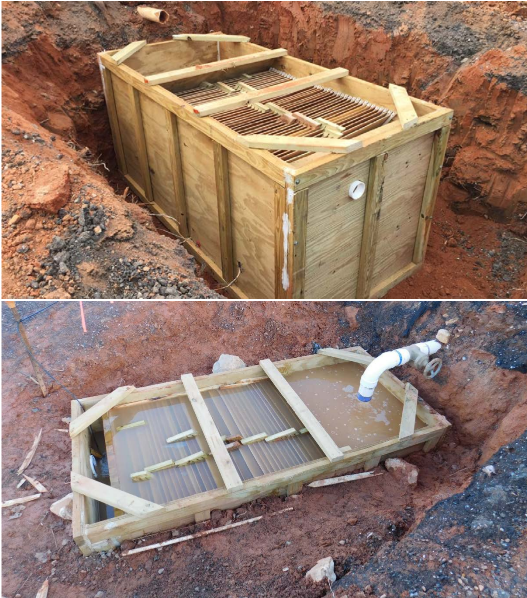
Figure 4.11: Completed small-scale lamella settler (SSLS) tank and unit in operation
