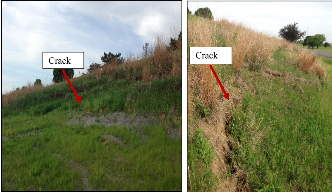
Figure 4.1 Failed slope at I-180 and Superior Street (2017)
