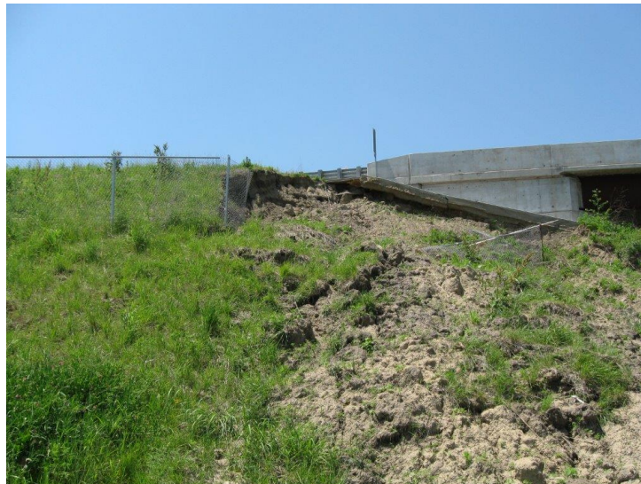
Figure 3.2 US-75, Mudslide (NDOR, 2015)
