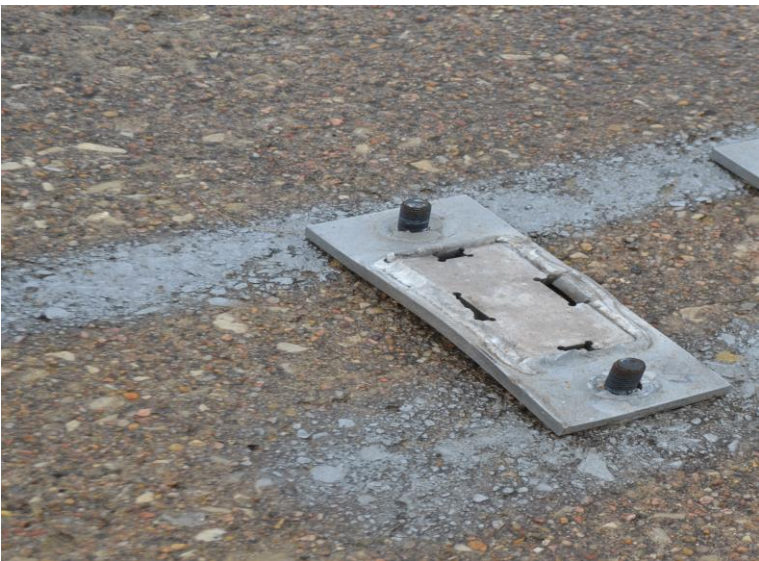
Figure 200. Panel No. 4 Damage, Test No. APR-2
