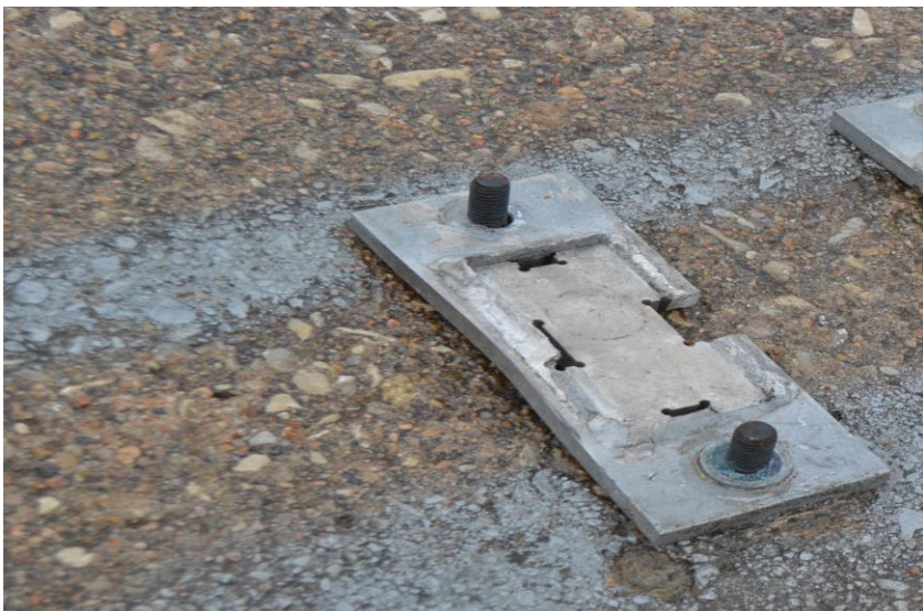
Figure 201. Panel No. 5 Damage, Test No. APR-2
