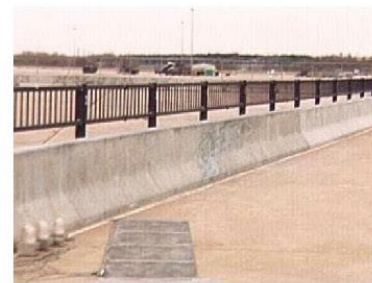
Figure 4. Concrete Traffic/Pedestrian Rail
