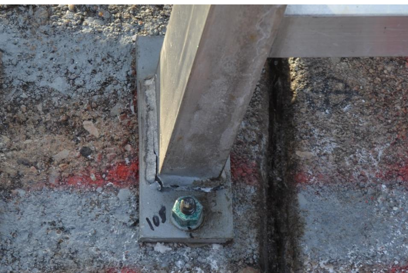
Figure 206. Panel No. 10 Damage, Test No. APR-2
