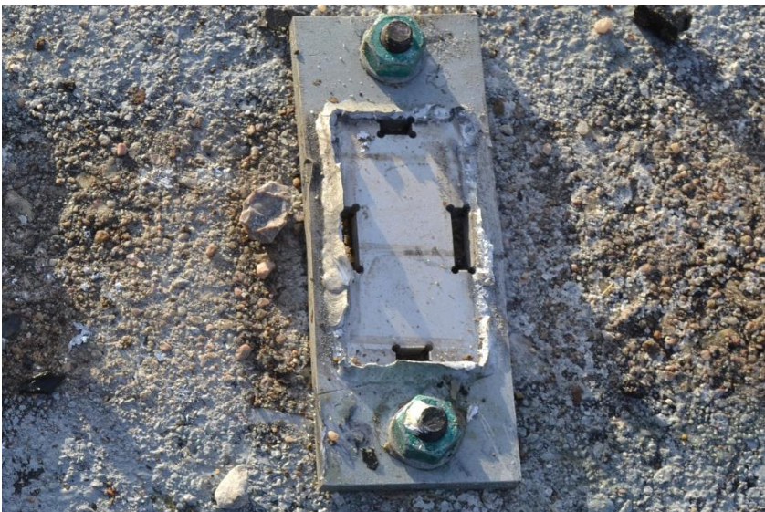
Figure 204. Panel No. 8 Damage, Test No. APR-2
