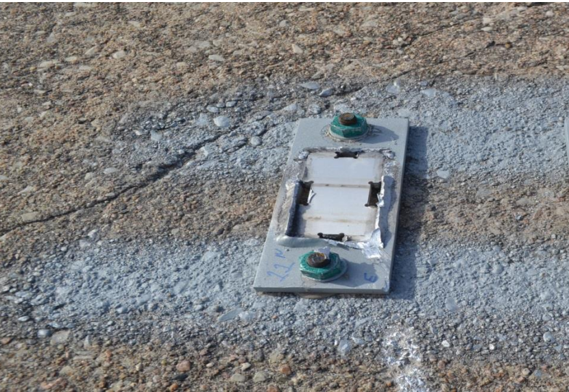
Figure 182. Panel No. 11 Damage, Test No. APR-1
