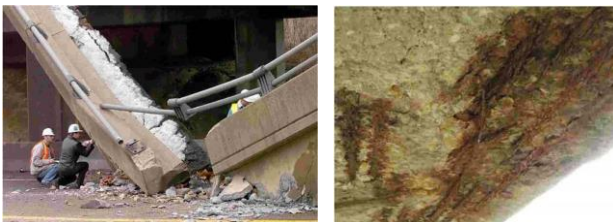
(a) Collapsed I-70 Lake View Drive Bridge, Pittsburgh, PA (b) Corrosion of the bridge
