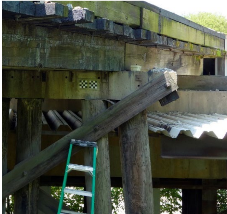
Figure 6.21 Sensors and target on the pier
