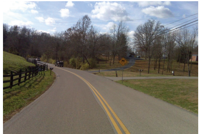
KYTC installed high friction surface treatments at locations with a history of wet roadway departure crashes.
