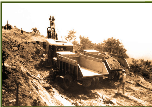
Excavation work on the Blue Ridge Parkway, shown here, included a crew drilling holes for explosives used to break up rock, while a diesel-powered shovel loaded earth into dump trucks.
