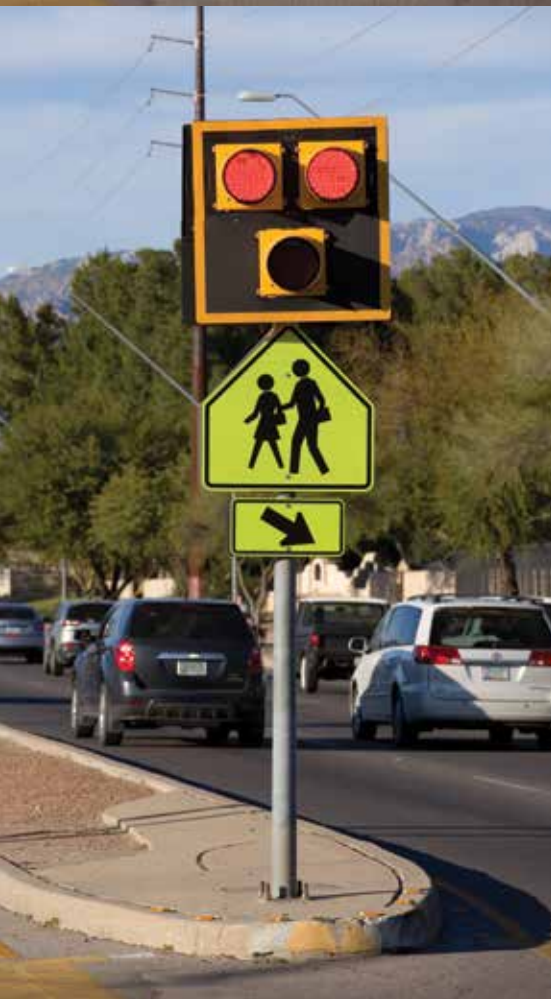
These two PHB indications show steady red, so drivers must stop and remain stopped. Photo: Martha Lochert Photography.
