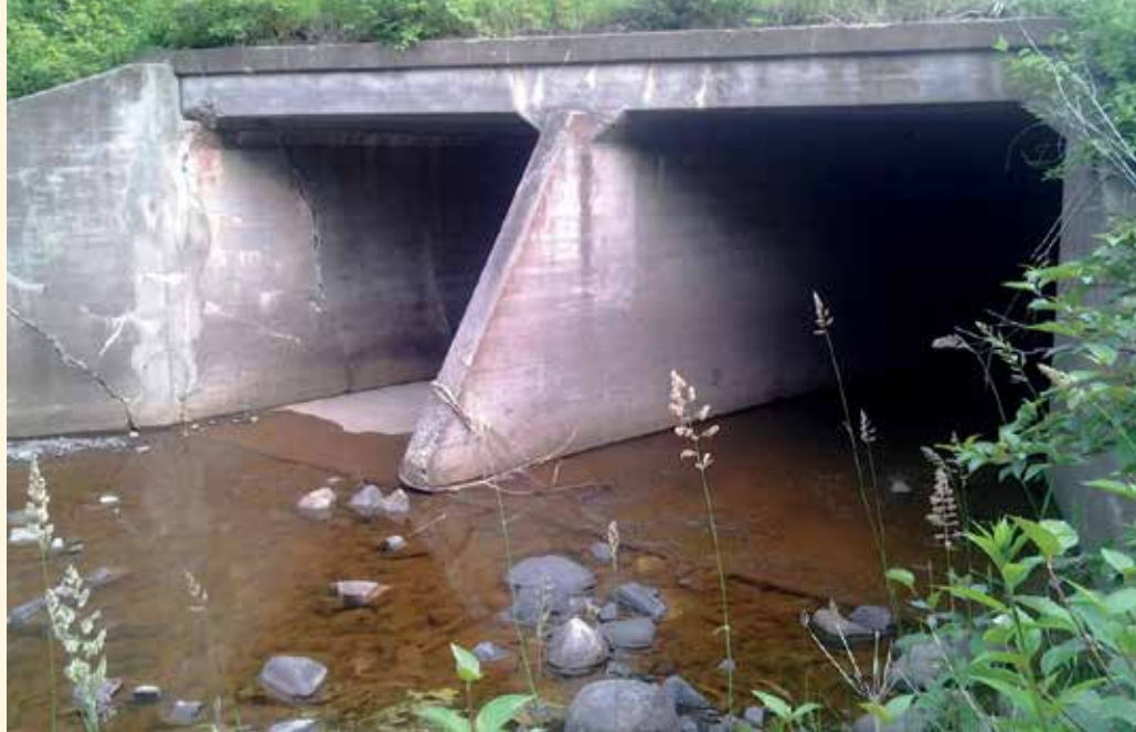
For culvert 5648, shown here, which carries MN-61 over Silver Creek in Minnesota's Arrowhead Region, the State used input from climate models indicating that a slightly larger replacement structure would be more cost effective in the long term. Photo: MnDOT.
