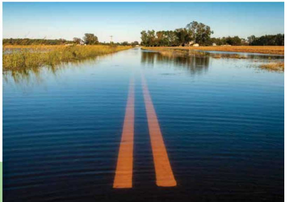
Shown is a flooded road in North Carolina. This road could be raised to possibly increase its resilience. Photo: © NikonShutterman, Getty Images.
