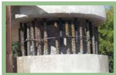
Shown is the connection of a new precast pier cap to an existing column prior to placement of the UHPC. Photo: Lafarge.
