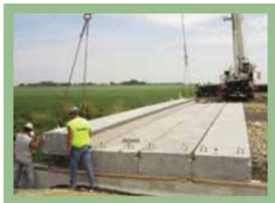
Shown here are four adjacent precast box girders that will be connected using UHPC. Photo: Eric Steinberg.
