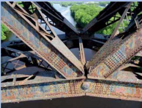
The drone proved to provide the level of detail needed to detect defects. In fact, the elements that are difficult to access through traditional methods were readily visible using the unmanned aircraft. Photo: Minnesota Department of Transportation.
