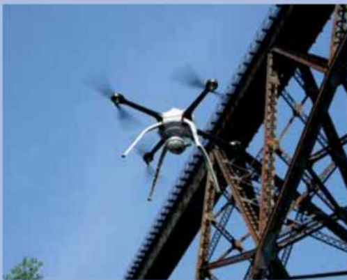
The Minnesota Department of Transportation used this unmanned aircraft to test the drone's inspection capabilities on the Arcola Bridge near Crystal Bay, MN. Typically, this bridge is inspected using rope access because of its height. Photo: Minnesota Department of Transportation.
