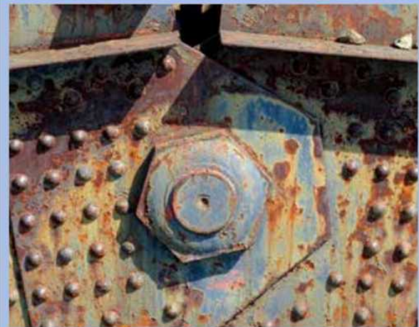
The zoom lens on the drone's camera captured a high level of detail without having to position the unmanned aircraft too close to the bridge. Photo: Minnesota Department of Transportation.
