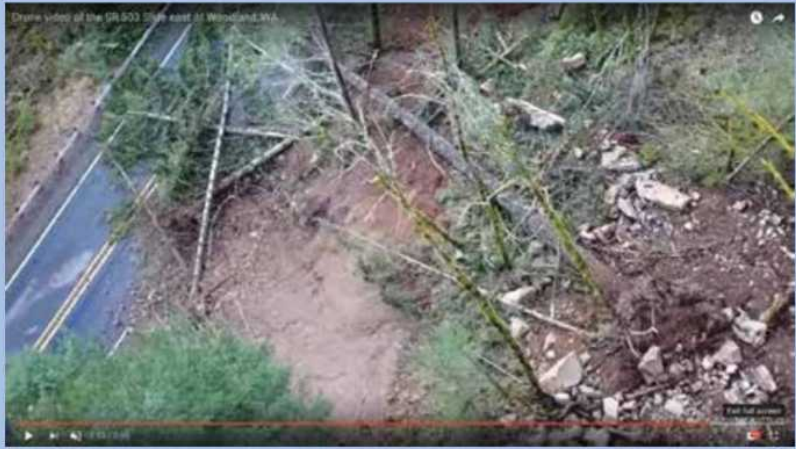
The Washington State Department of Transportation used a drone to capture video footage for this up-close view of a slope on State Route 503 that requires stabilization. Photo: Washington State Department of Transportation.
