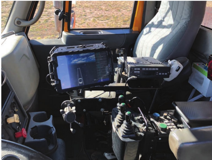
This human-machine interface (a tablet computer) is installed in a WYDOT snowplow. Photo: WYDOT.
