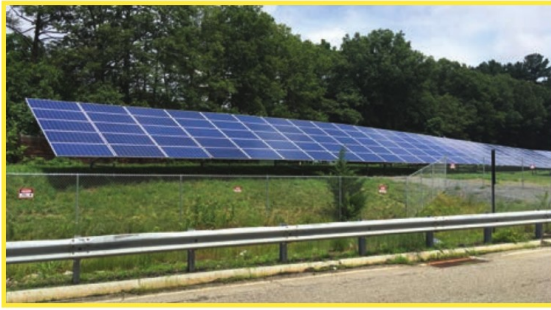
These solar panels are located at the Framingham Service Plaza on I-90 in Massachusetts.
