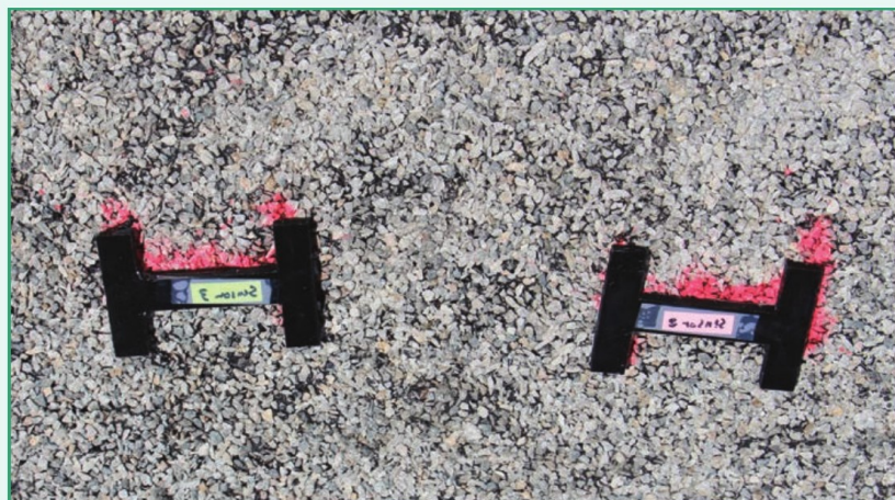
These packaged PFG sensor prototypes are being installed at the accelerated pavement testing facility at The French Institute of Science and Technology for Transport, Spatial Planning, Development and Networks (IFSTTAR) in Nantes, France. The sensors were installed by the Michigan State University and Washington University research team in collaboration with researchers at IFSTTAR. Photo: Nizar Lajnef, Michigan State University.
