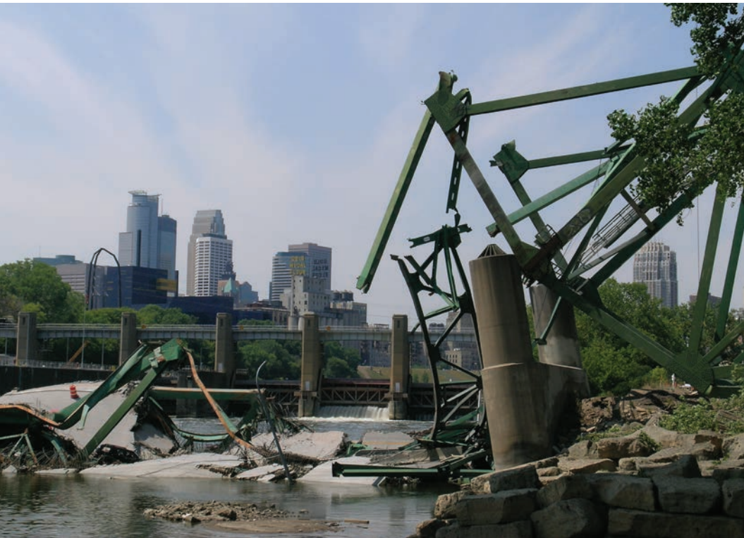
In his leadership roles, Wright faced a lot of challenges. One of the most notable was FHWA's response to the I-35W bridge collapse in Minneapolis, MN, in August 2007. Photo: FHWA.
