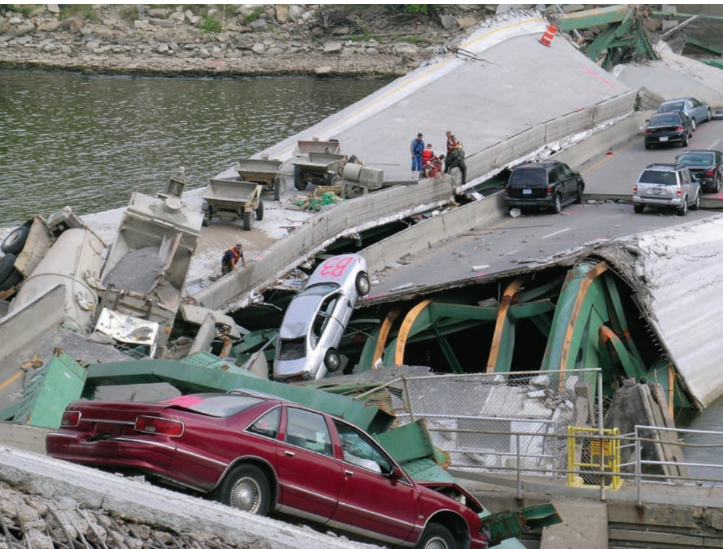
Under Wright's leadership, FHWA responded to the I-35W bridge collapse by taking a coordinating role, bringing together stakeholders. Photo: FHWA.
