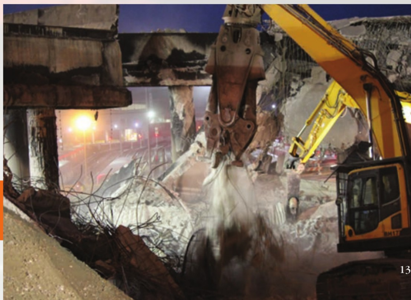
Demolition of the damaged spans began just hours after the fire was extinguished. © GDOT.
