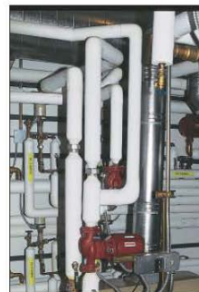
The CR5000 can monitor and control pumps, fans, and starter motors in an HVAC system.
