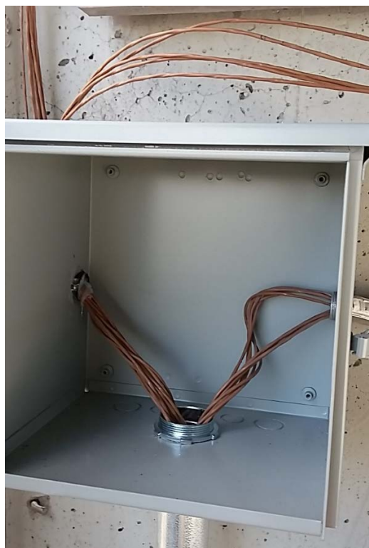
Figure 3.13 West column junction box
