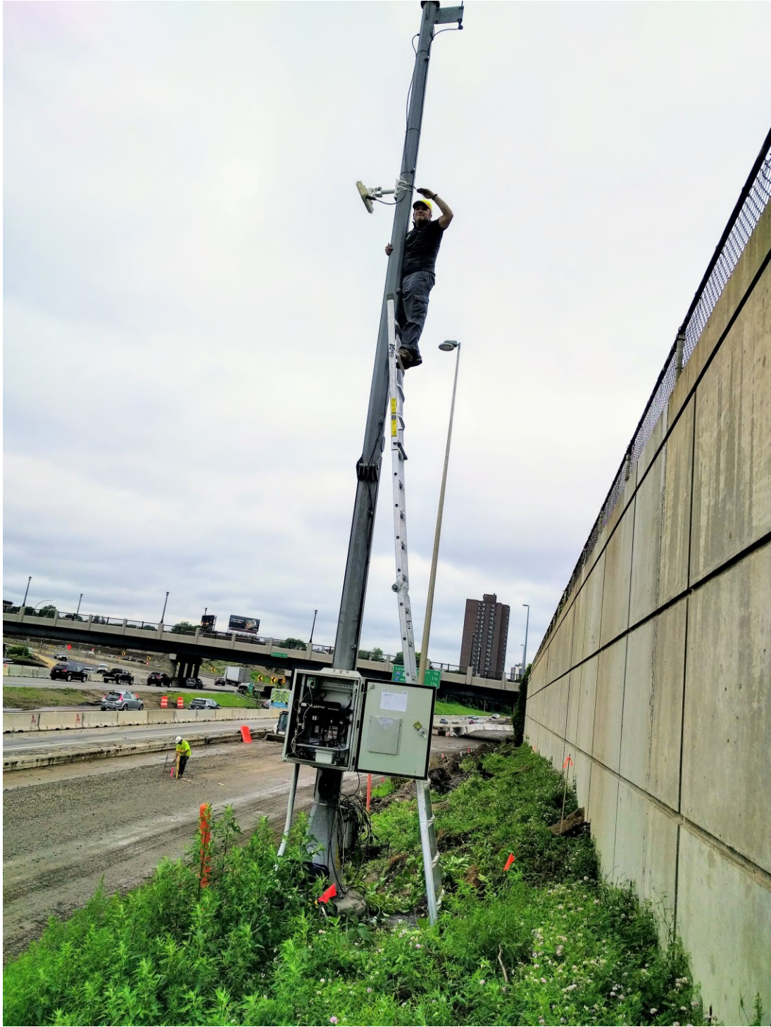
Figure 2.8 Retrieval of the Park Ave Sensor
