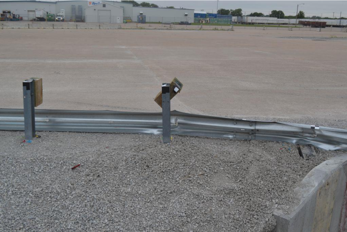
Figure 54. Damage Between Post Nos. 14 and 16, Test No. MGSL-1
