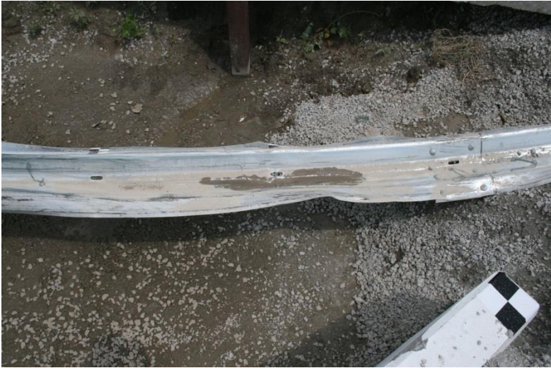
Figure 72. Damage Between Post Nos. 13 and 14, Test No. MGSL-2
