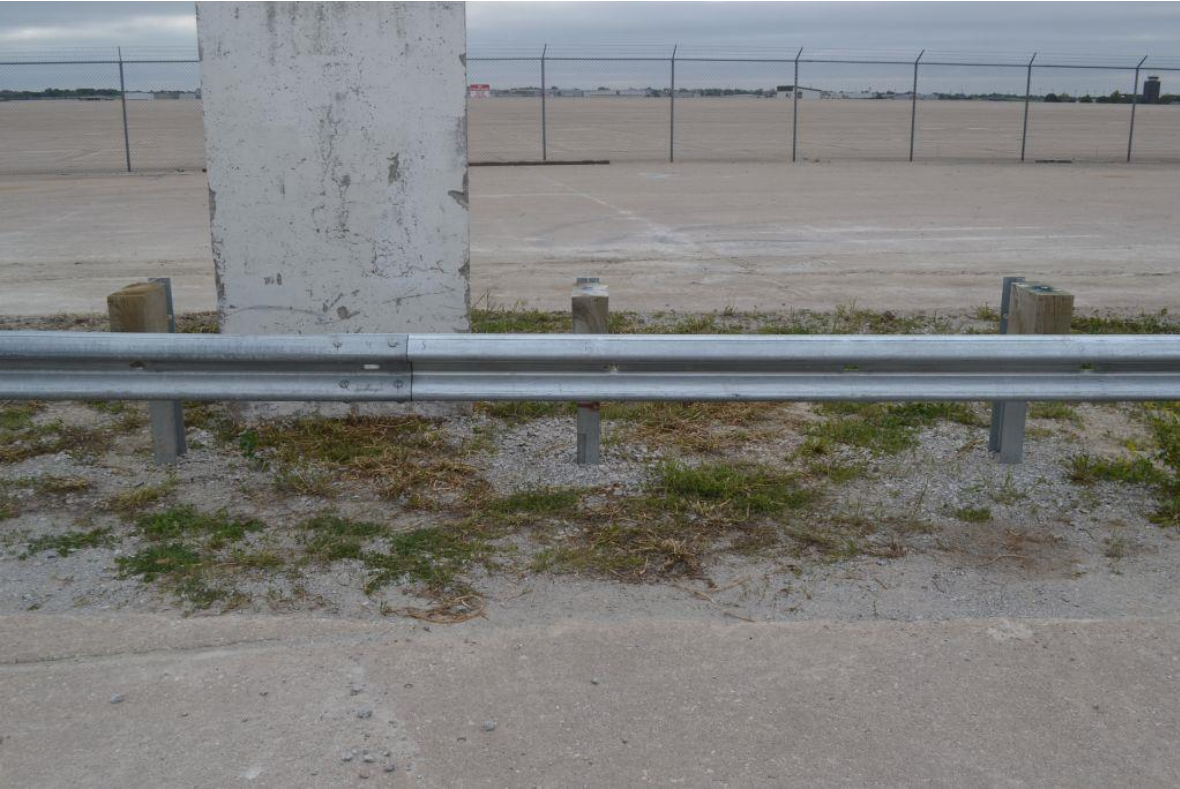
Figure 50. System Damage Between Post Nos. 3 and 9, Test No. MGSL-1
