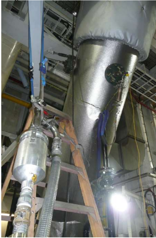
Sampling ports before Scrubber
