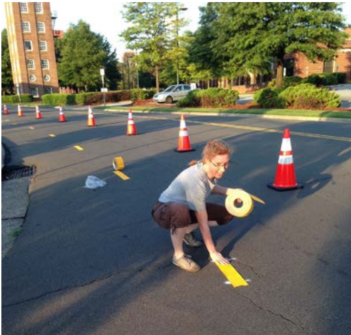
Figure 4: Striping roads for road safety. (Image courtesy of the city of Durham)
