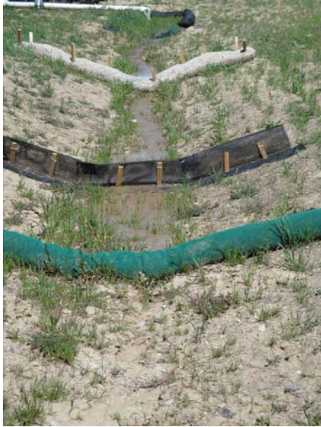
Check dams, an example of a sediment control technique, displayed at the Colorado DOT's (CDOT) Best Management Practices training facility. (Courtesy of FHWA)
