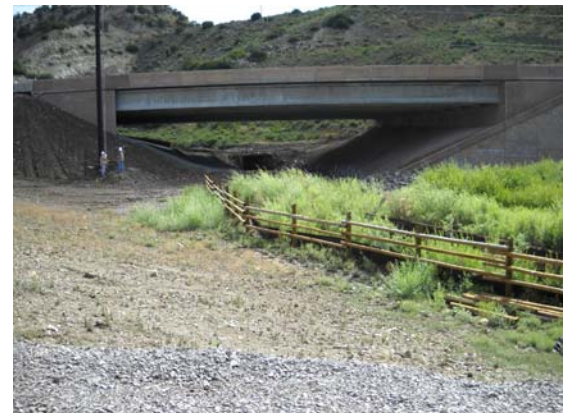
Mile-point 203 is the location of a road-widening and bridge-construction project along US 6 in Utah. The project is part of the Wildlife Coordination Committee's efforts to develop wildlife mitigation measures. (Courtesy of Wildlife Coordinating Committee)
