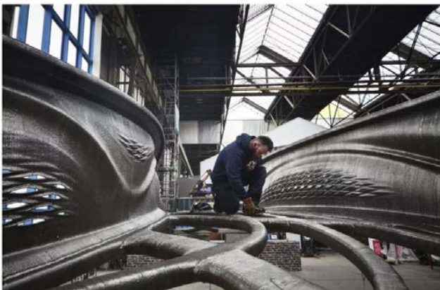
A steel deck will cover the curved supports on the bottom of the bridge Photo: Adriaan de Groot
