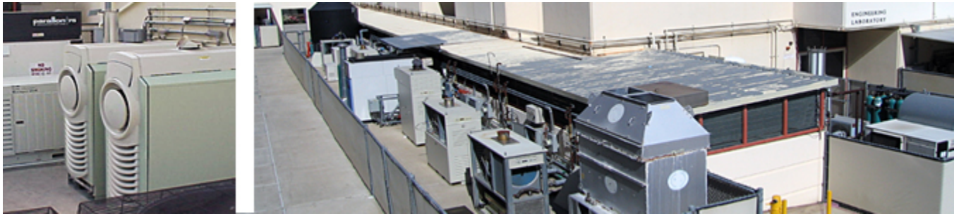
Figure 2. Photographs of the Distributed Generation Testbed of the NFCRC
