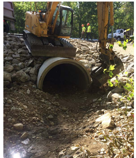
A culvert is constructed in Maine following the programmatic consultation. (Image courtesy of MaineDOT)
