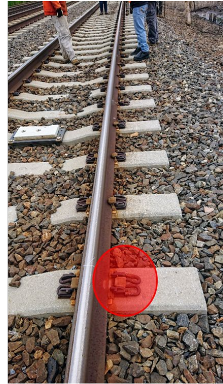
Figure 69 – Deliberate Changes to Fastener Conditions in the Field (missing on the left and loose on the right)
