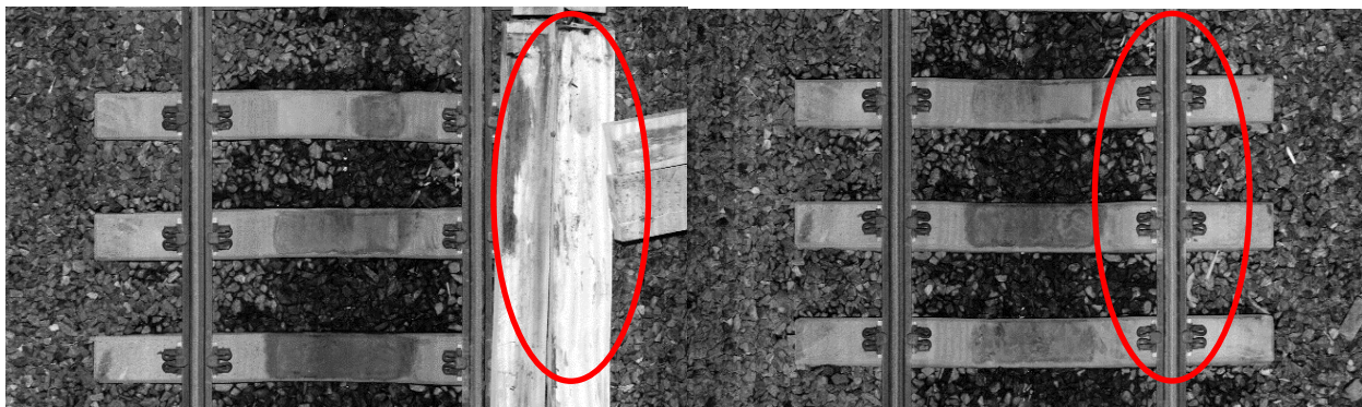
Figure 28 – Unplanned Removal of Wooden Planks (D2R1 on left and D2R2 on right)
