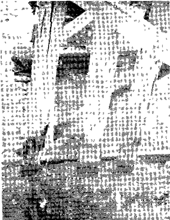
Plate 2. Showing failure of the east outside batter pile of an original full-pile bent because of decay; also shows longitudinal split.
