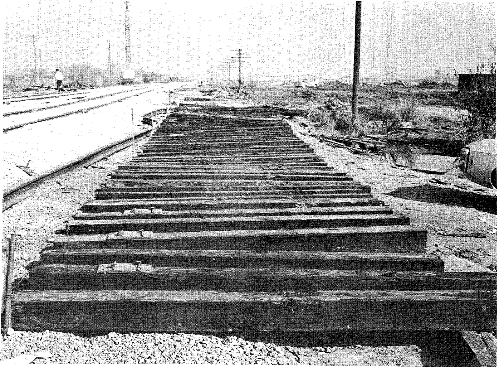
Figure 10 - View looking north showing switch ties reassembled after the accident. Tie at the bottom of photograph is the first headblock tie. Rail to the left of switch ties is the east rail repositioned following the accident.
