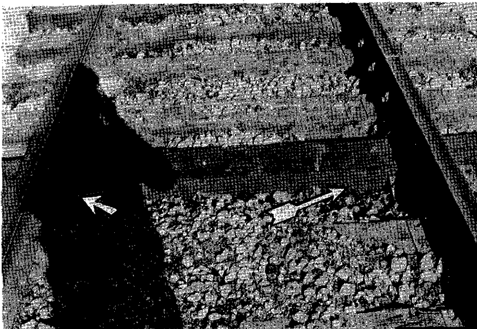
Figure 3.—Unspiked new crosstie about 300 feet south of the point of derailment.
