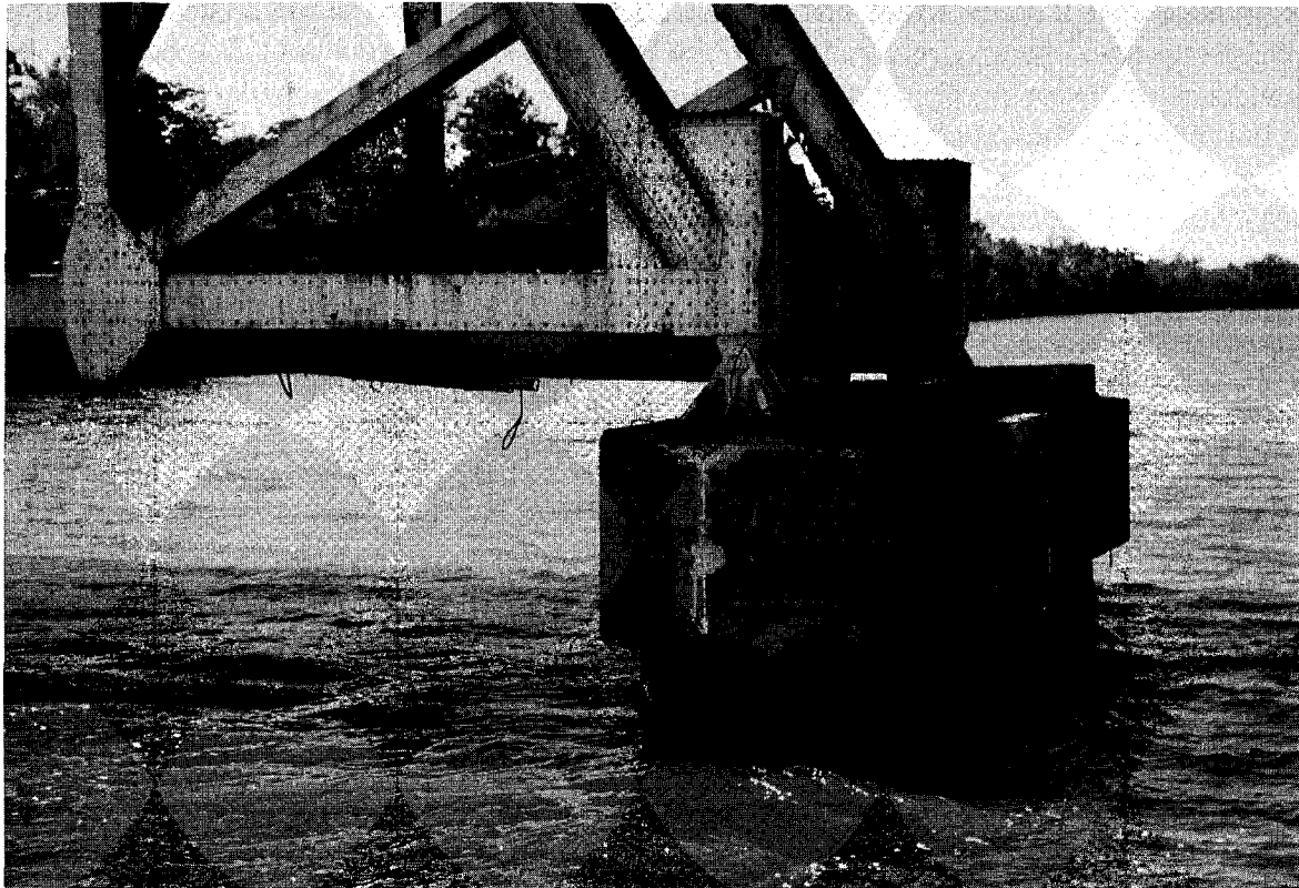
Figure 7.--Collision marks on Big Bayou Canot bridge.
