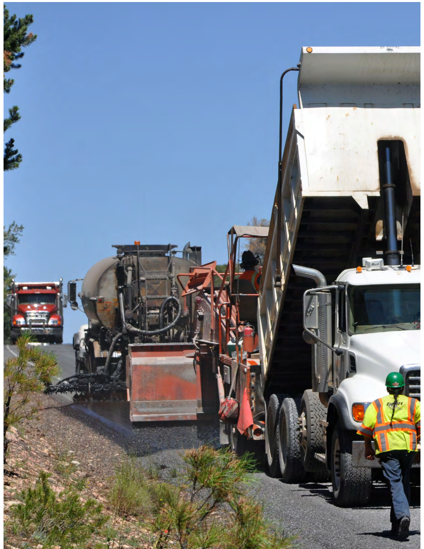
Advanced, proven preservation practices can help extend the overall service life of pavements.
