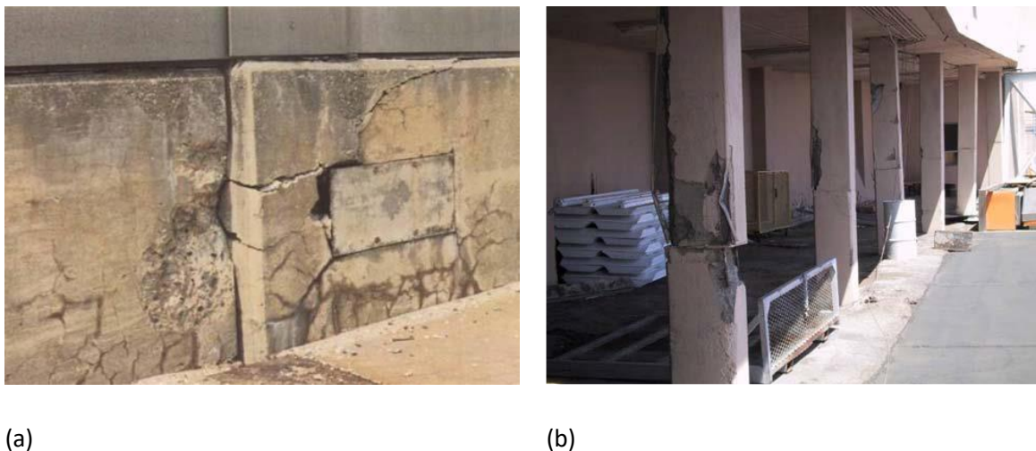
Figure 1.8: Structural distress due to ASR, (a) Relative movement of abutting sections of parapet wall in a bridge structure affected by ASR (from Stark, 1991), (b) Expansion of concrete pavement due to ASR (overlaid with asphalt), which pushes against the adjacent building foundation causing shearing of concrete columns (from Thomas et al., 2013).
