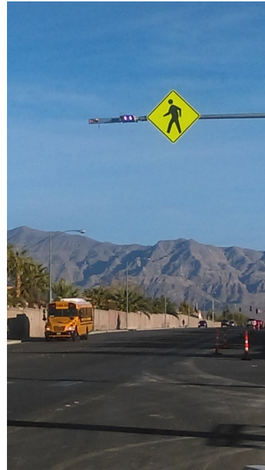
(d) LED light is operational
