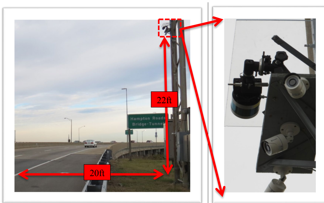
Figure 1 LIDAR and surveillance cameras mounted on the gantry pole before the Willoughby Bridge
