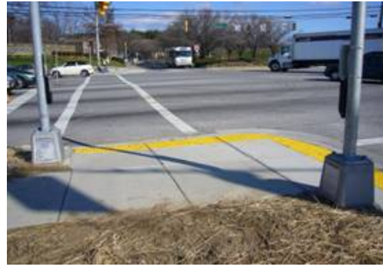
Figure 1: Pushbutton-integrated APS installed on separated poles, beside crosswalk each serves
