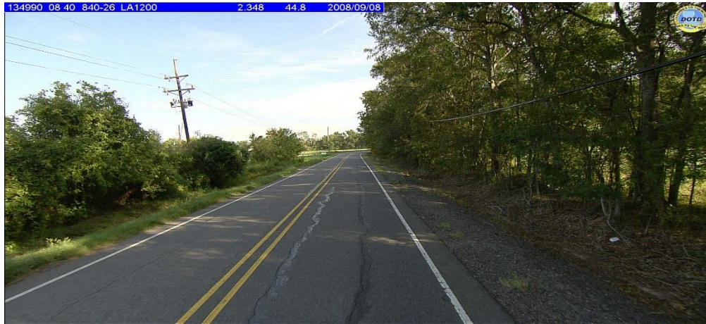
Figure 1 Longitudinal cracks: LA 1200: CSLM 2.348
