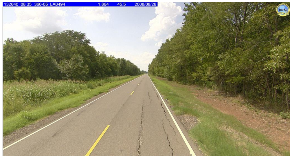
Figure 2 Multiple longitudinal cracks: La 494: CSLM 1.864
