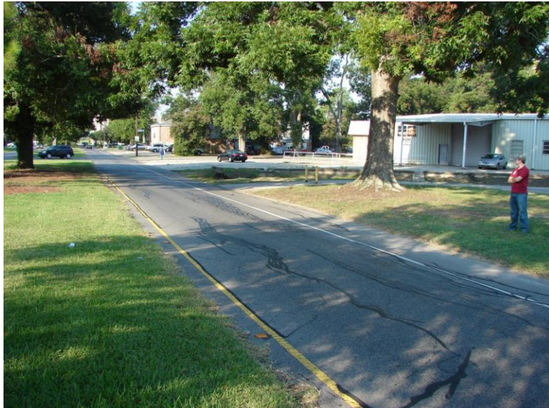
Figure 7 Multiple longitudinal cracks and subsidence: West Parker Ave. near LTRC
