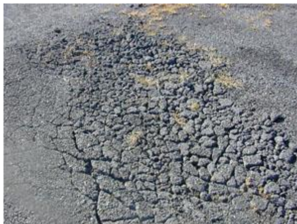
Figure 4 Alligator cracking in AC surface
