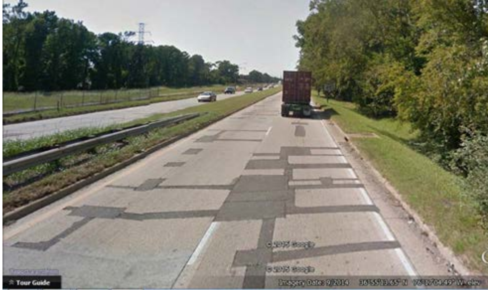
Figure 3. Existing SR 406: CRCP in Poor Condition. CRCP = continuously reinforced concrete pavement.
