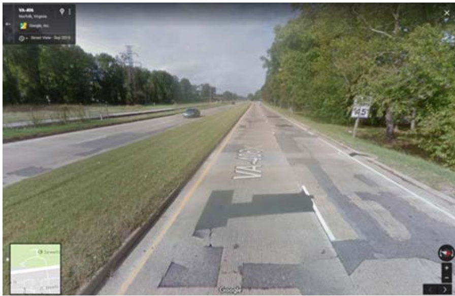
Figure 2. Existing SR 406: CRCP in Poor Condition. CRCP = continuously reinforced concrete pavement.
