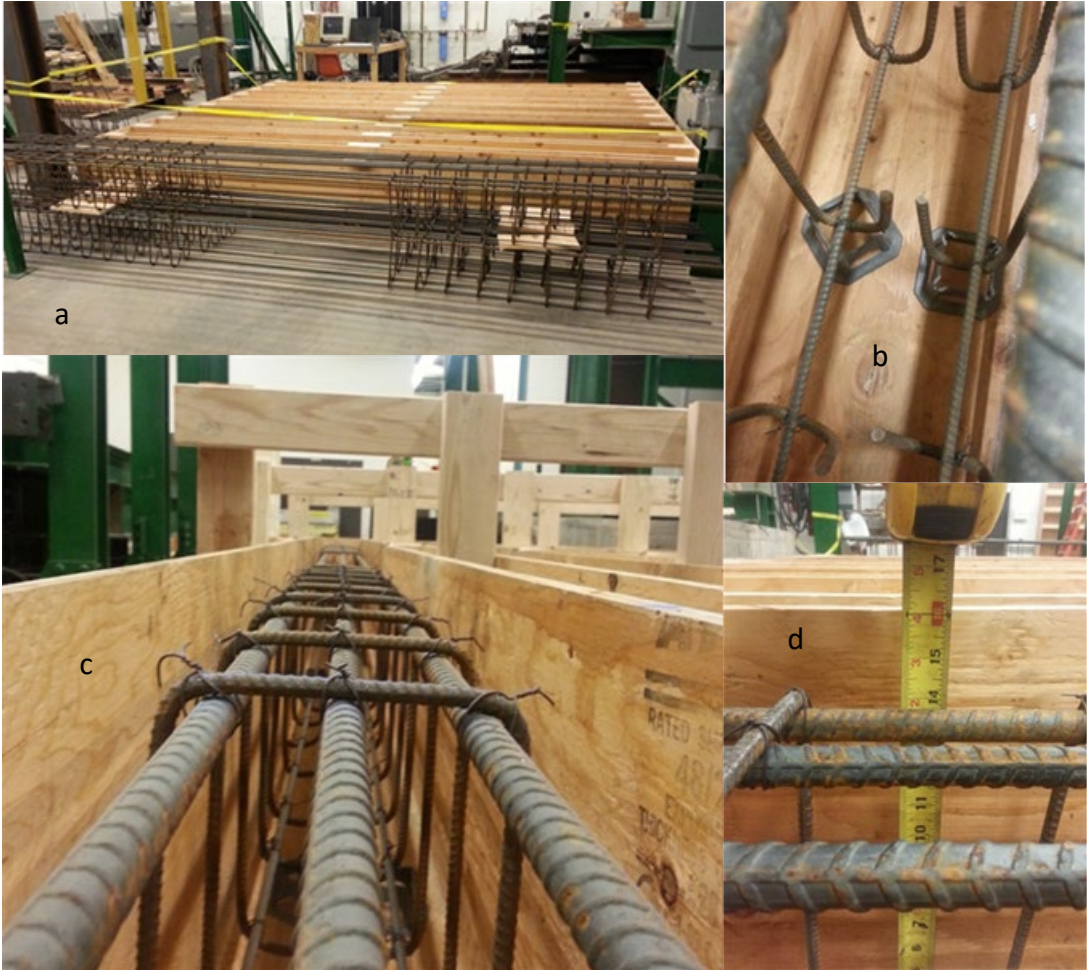
Figure 2.12 a) Rebar cages, b) 40mm plastic rebar chairs, c) position of rebar cage in form, d) depth of tensile reinforcement once supported on 40mm rebar chairs
