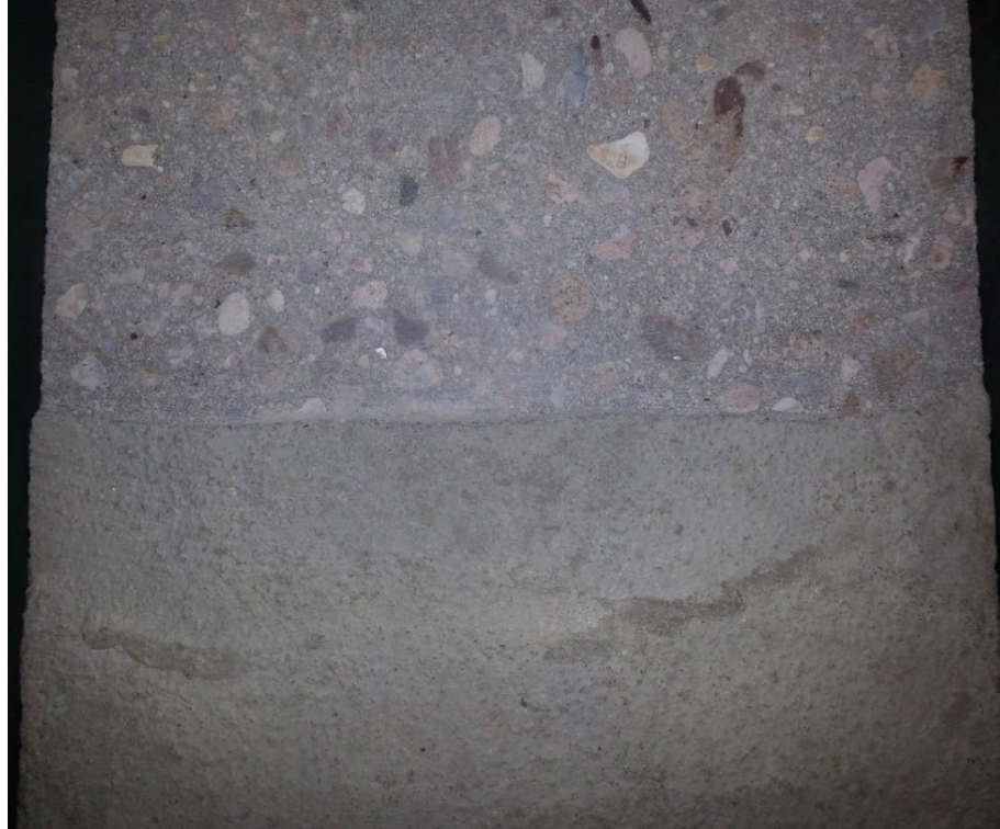
Figure 2.14 Concrete surface, top; removed laitance layer exposing aggregate, bottom; concrete surface left by finishing of wet concrete
