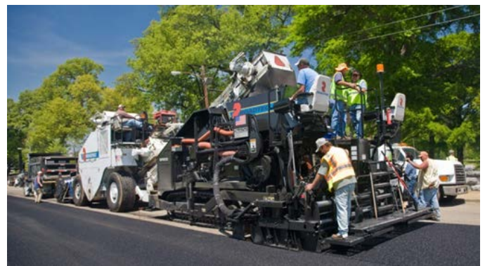
A construction crew conducts paving operations on a roadway. Photo courtesy of Transtec, Inc.
