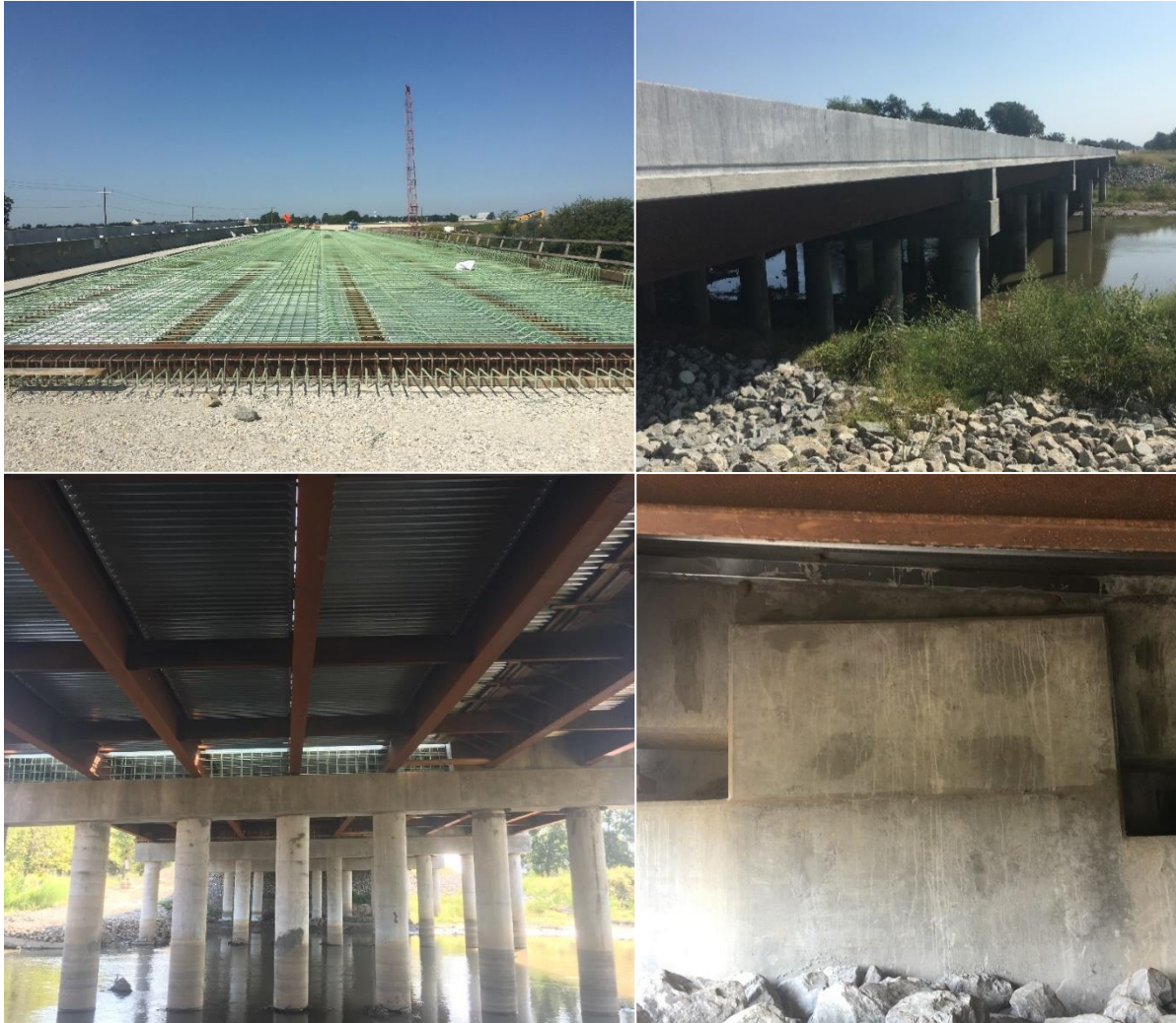
Figure 5. 2: Monette Bypass Bridge construction. Top Left – Second phase of deck construction. Top Right – South side of bridge (looking East bound) crossing Cockle Burr Slough. Bottom Left – View of steel girders and pile bent 3. Bottom Right – View of restrainer block on bent 1.
