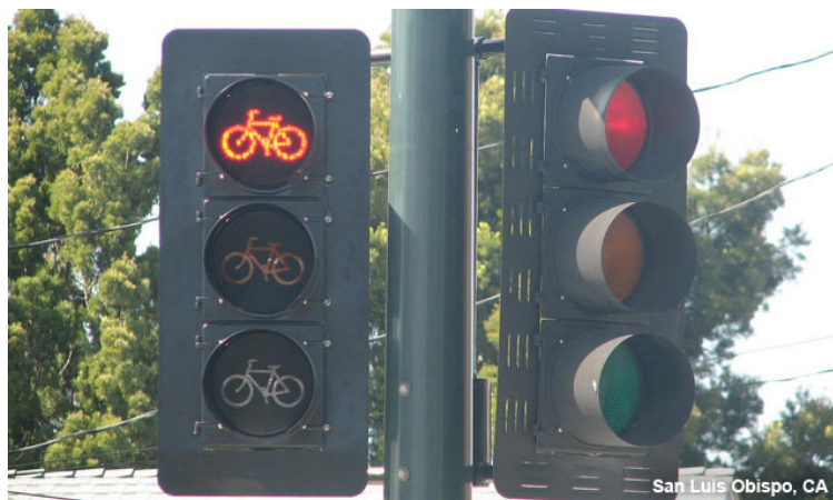
Figure 4- Typical bicycle signal head
